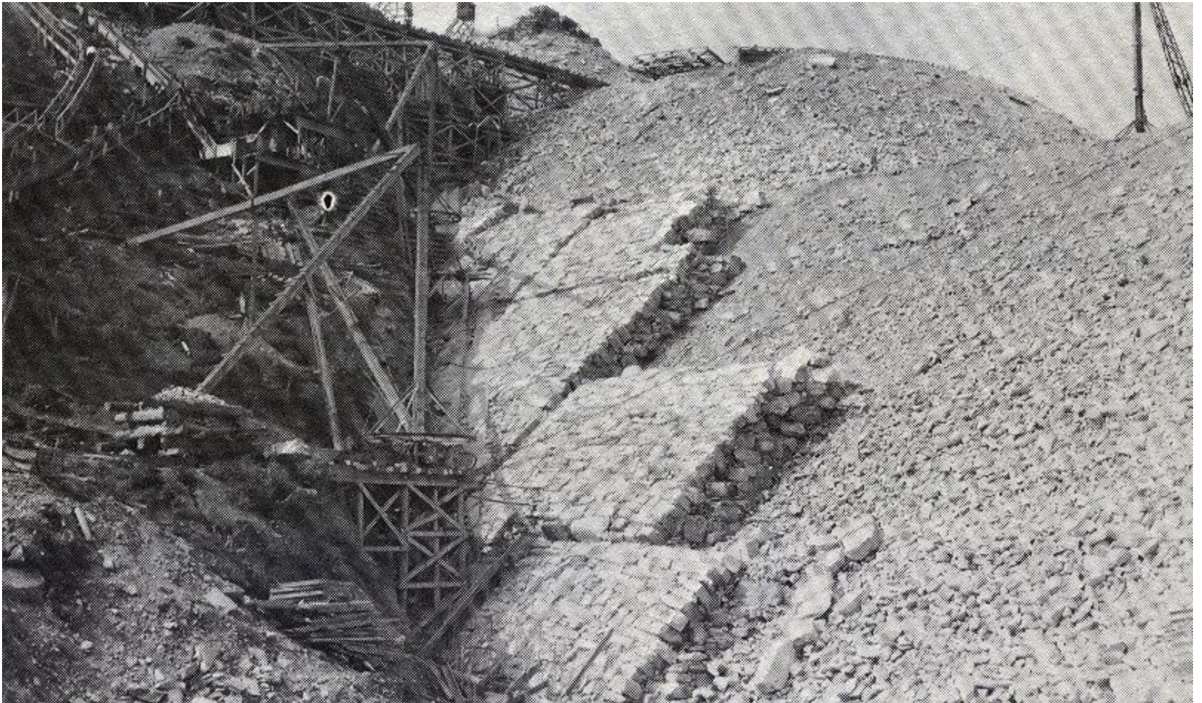
Derrik-Laid Masonry on Fill (Note H&V Joint Recesses) (Schmidt, L. A., jr, "DIX RIVER DAM", Symposium on Rockfill Dams, 1960)
